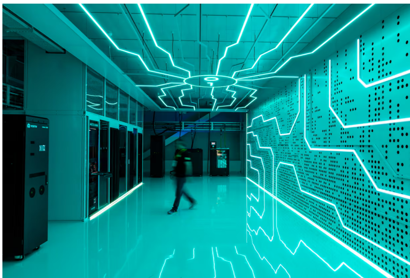
Liquid-cooled servers at the Global Switch data centre, London. Photograph: Bloomberg/Getty Images
